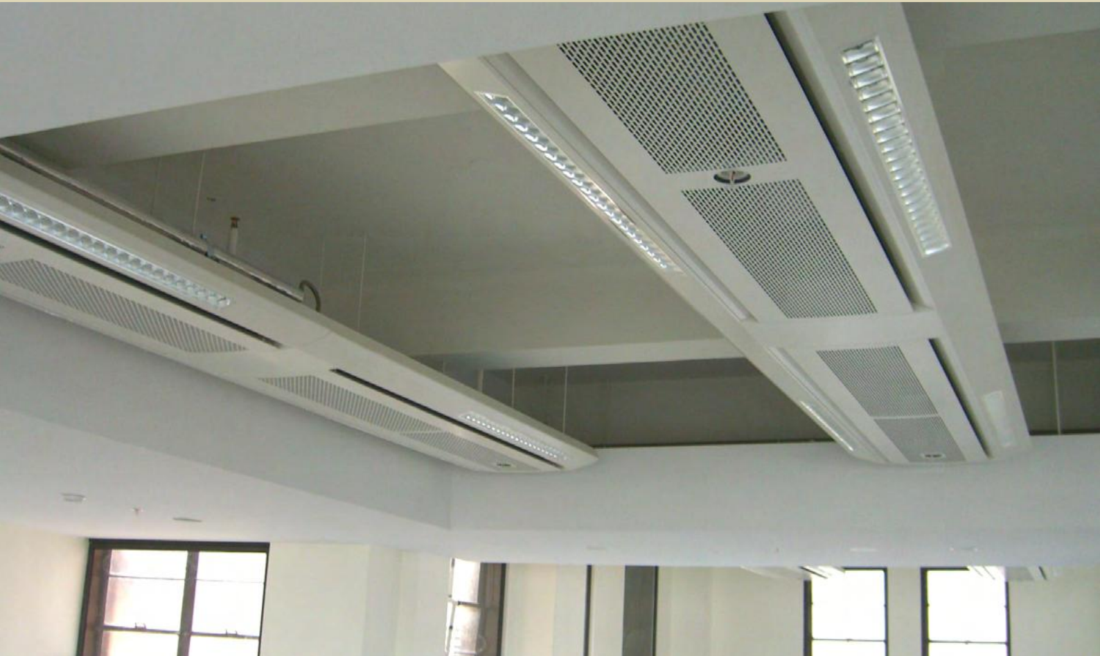
Transport House original installation - 2008
