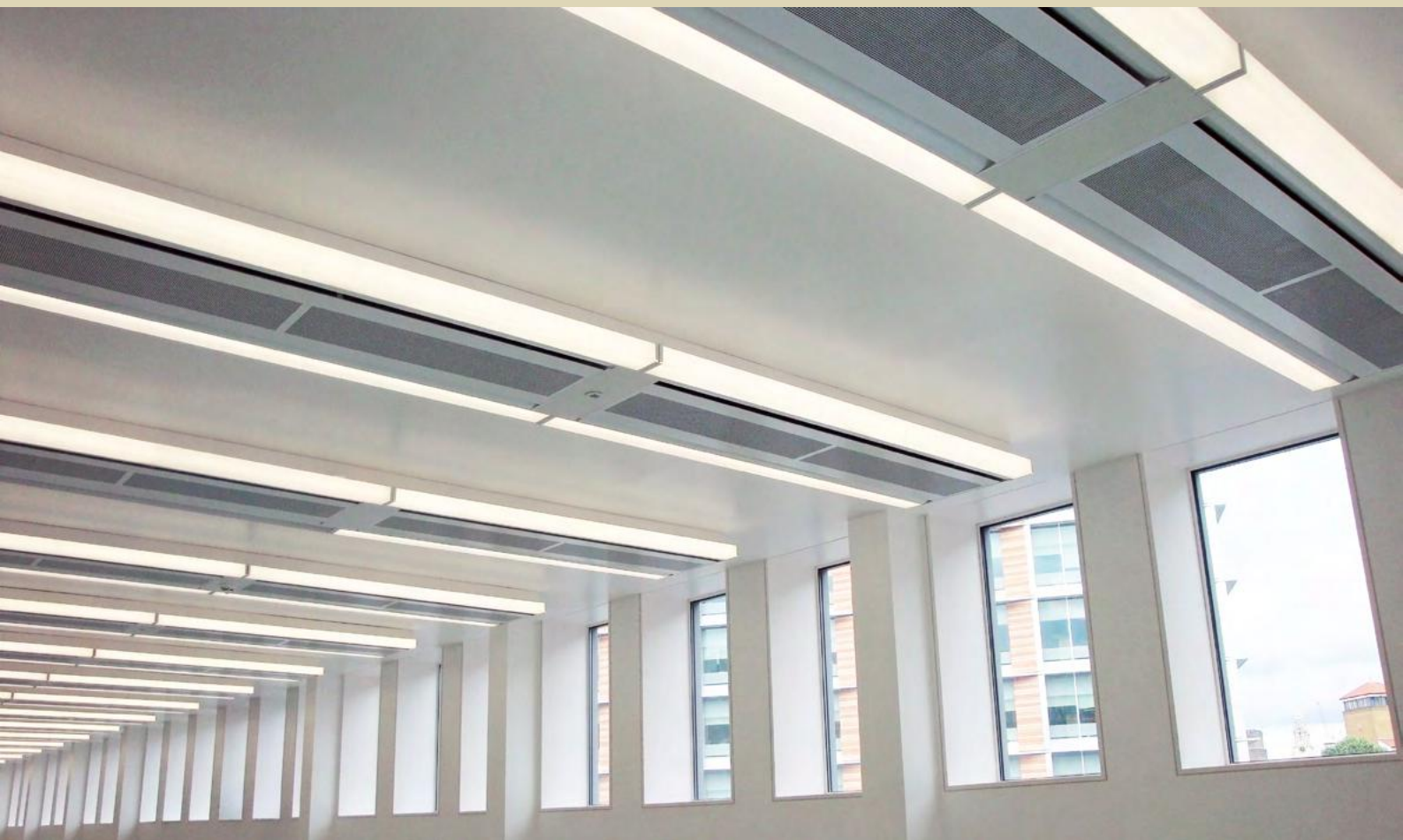
65 Southwark Street original installation - 2012
