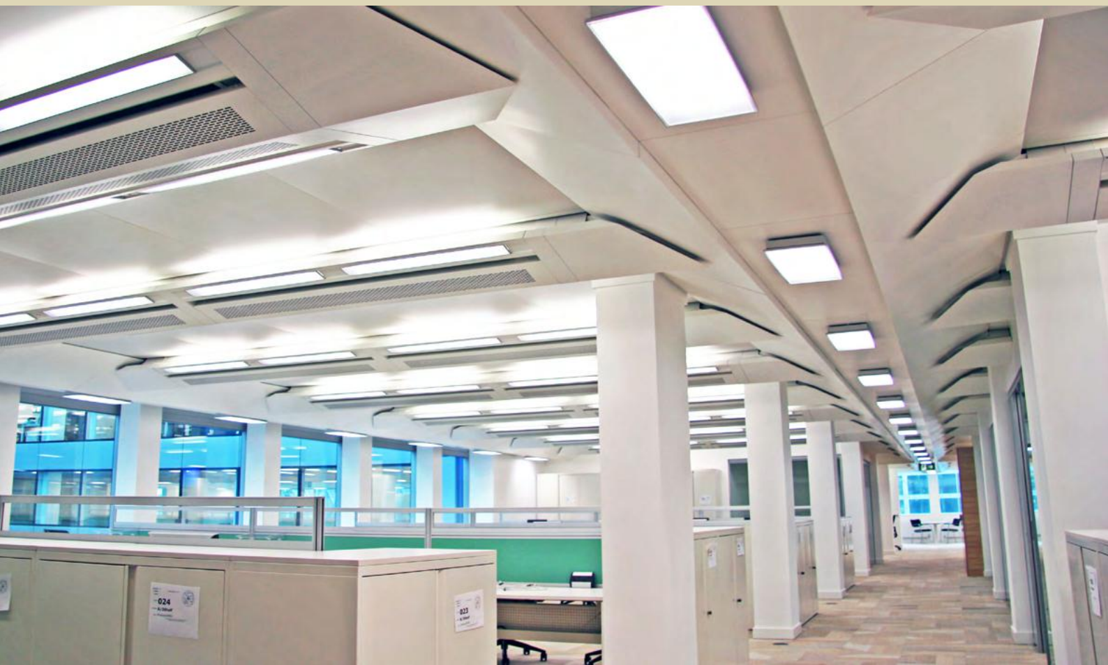
55 Baker Street original installation - 2007
